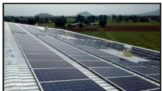
85 KW Parmeshwar Cold Storage, Kheralu, Mehsana, Gujarat
