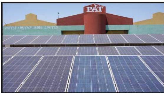
130 KW Patel Airtemp, Santej GIDC Ahmedabad, Gujarat
