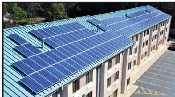
57.6 KW ABVI Hotel, 2185 Mt Zion Pkwy, Morrow, GA USA
